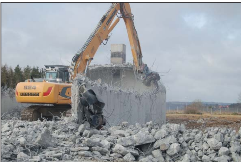
German contractors BG Werning/Weihrauch use heavy equipment to demolish concrete portions of an old bunker at Urtas, Germany. The concrete is crushed into smaller particles that will be completely recycled.
