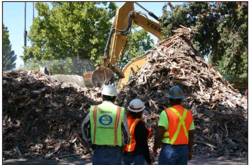
Gregorio Pena, Ferma Corp., left, Mindy Shelton, Huntsville Center, and Milton Dozier, Bhate Associates, watch a backhoe crunch up debris at a facilities removal project at Moffett Field, Calif.
