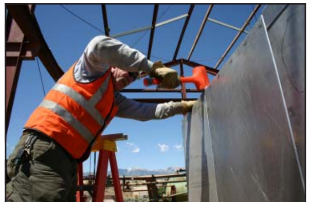
Bill Menzl, PIKA International, seats a panel, which is part of the enclosure being built around equipment at Tooele Army Depot. The enclosure is part of a Thermal Convection System that will be used to burn off trace explosive residue so the equipment can be cut up and recycled as part of a Facilities Reduction Program project at Tooele, near Salt Lake City, Utah.
